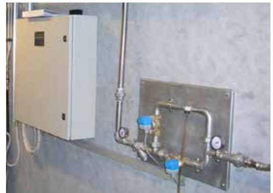
Control Board Automatic CIP cleaning unit.
