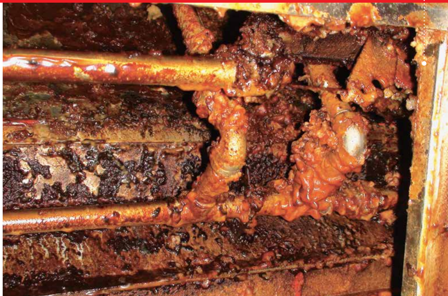
Hood without JIMCO Technology - Not cleaned for 6 months
