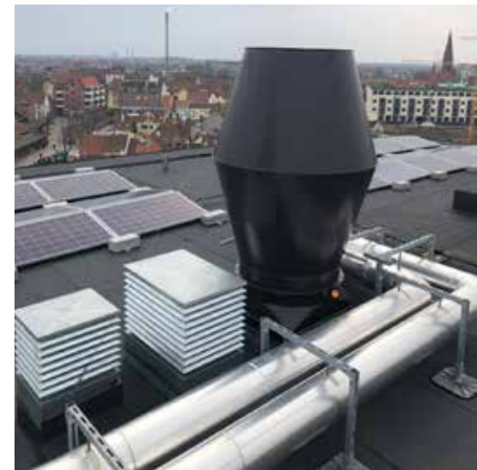
Air outlet from the kitchen
