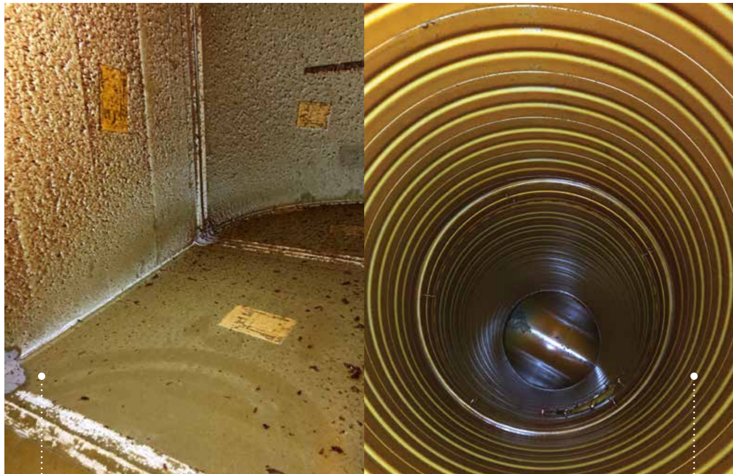
Grill duct with JIMCO Technology - Not cleaned for 60 months
